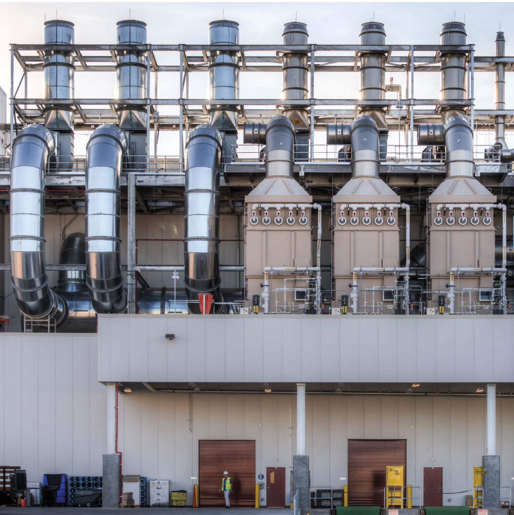
Emissions abatement systems and cooling towers benefit from recycled water with improved efficiency, lower operating costs and cleaner air emissions. Photo: George Tenney
