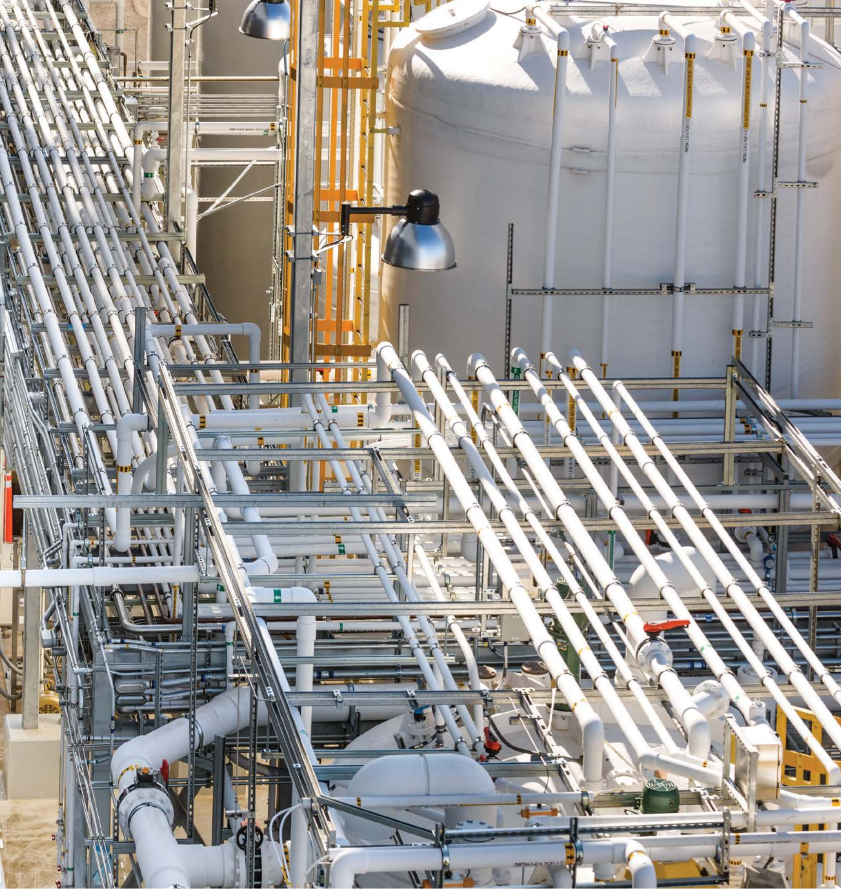
At Intel's manufacturing facilities, gray water from reverse-osmosis systems is reclaimed for landscaping irrigation and toilets, increasing total cycles of on-site water reuse. Photo: George Tenney
